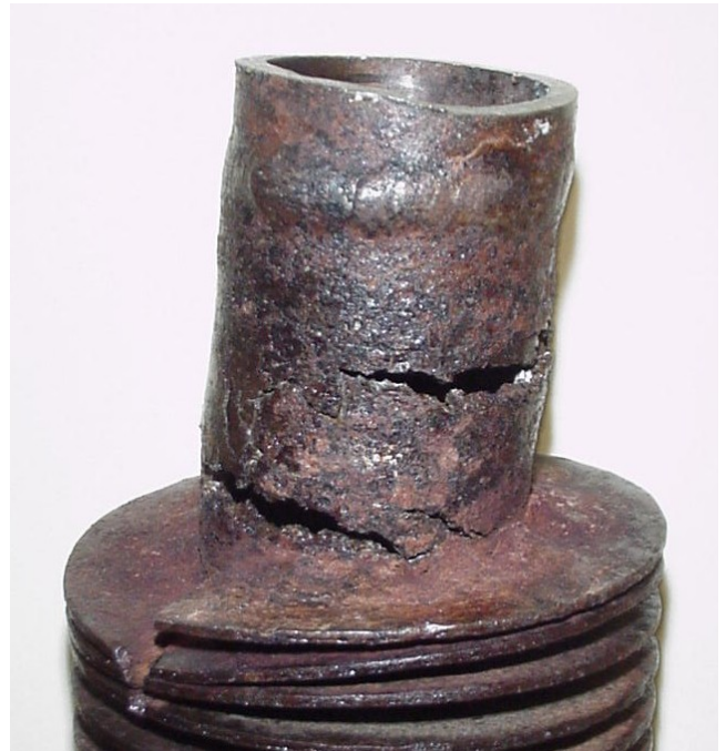
Severe SCC damage to a stainless steel superheater tube
