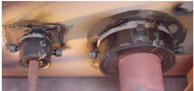
Superheater floor penetrations for drain and crossover pipes
